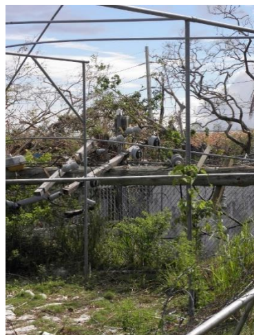
The high voltage post
